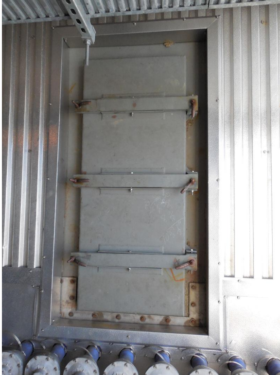
Walk in Plenum with insulated entry door
