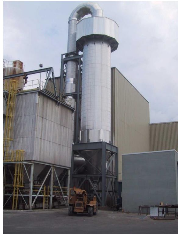
Spray Dryer/Absorber and Fabric Filter
