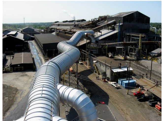
18 Ft. Diameter Melt Shop Ventilation
