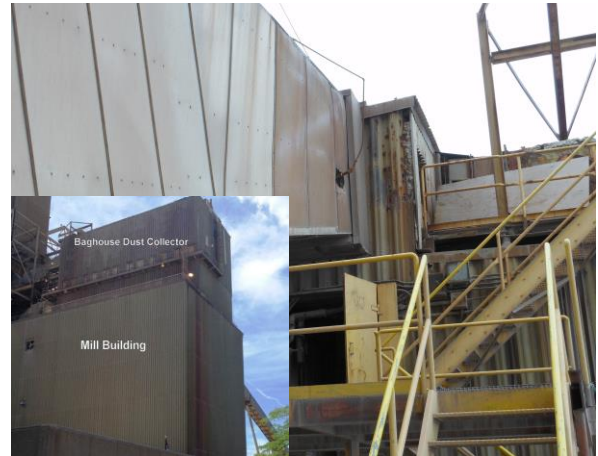
Deteriorating Kiln/Raw Mill Baghouse
